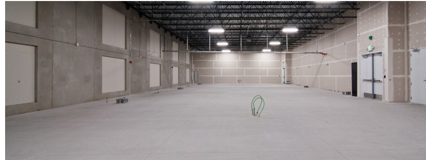
A future data center floor.
